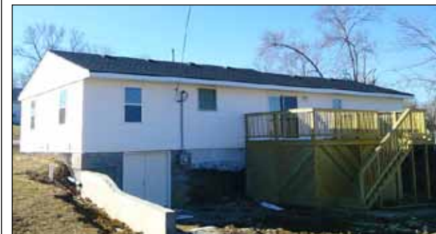
Brian Carter added two nice decks to his recently remodeled home on Vandivert Street in Bethany.
